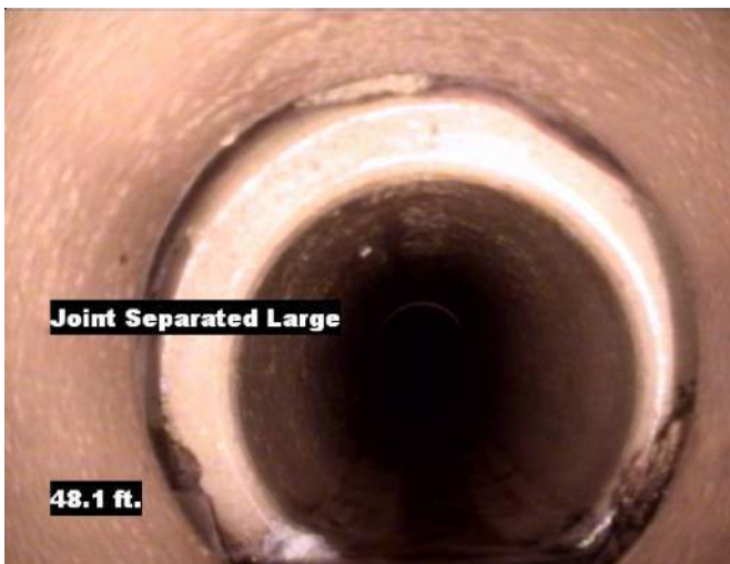
Joint Separated Large 48.1 ft. Distance: 48.1 ft. Grade: 2 Condition: Joint Separated Large Remarks: N/A
