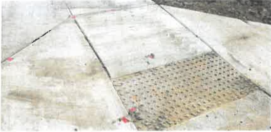
Image 39 (4208) – Chipped concrete, fly ash, and other debris imbedded in ramp – Clean up.
