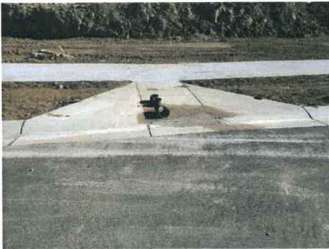
Image 1 – Ponding drainage - Remove/replace curb ramp & gutter. Cracks in sidewalk at top of ramp – Remove/replace
