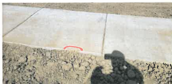
Image 23 (1711) – Chipped concrete – Monitor during warranty period. Revised July 27, 2020
