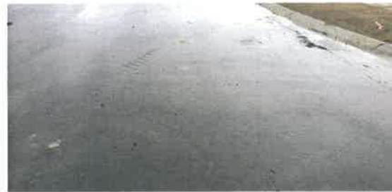
Image 50 (5458) – Gouged asphalt from equipment – Mill and overlay, monitor during warranty period.
