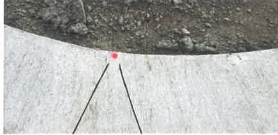
Image 40 (4230) – Saw line of control joint not completed to end of asphalt – Finish saw cut.
