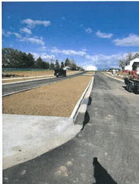
Image 2 – Ponding in curb and gutter – Remove/replace curb and gutter to achieve intended design drainage conveyance
