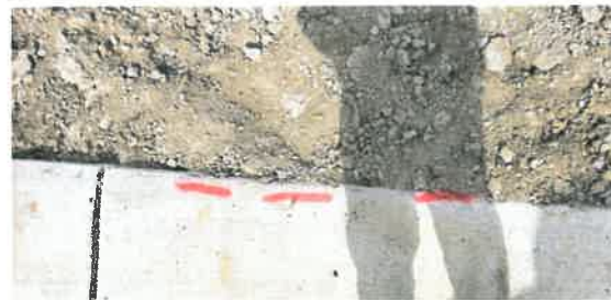
Image 24 (1725) – Chipped concrete – Monitor during warranty period. Revised July 27, 2020
