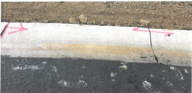
Image 43 (4508) – Ponding of surface drainage in gutter – Remove/replace curb and gutter to achieve proper drainage.
