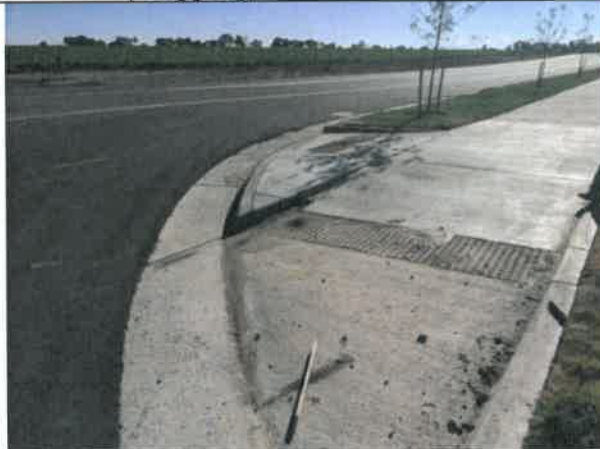
Image 11 – Concrete ramp with pointed curbs at WCR 5 and WCR 32 intersection to be monitored through warranty period.
