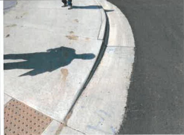
Image 12 – Curb ramp at WCR 5 and Kerry Street has settled causing a trip hazard.
