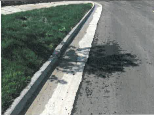
Image 9 – Poor workmanship, and flowline within WCR 5 north of Charbray Street pushes out into traffic.
