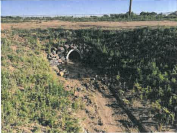
Image 9 – Swale elevations at the end of the riprap protection are set higher than riprap elevations, trapping water.
