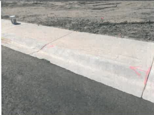
Image 11 – Paint markings direct contractor to remove excess asphalt and patch chipped concrete. Typical in site areas.
