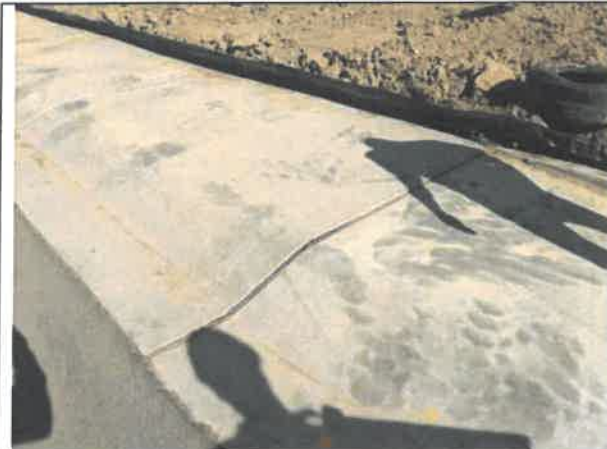
Image 3 – Scuffed concrete, typical in areas around site.
