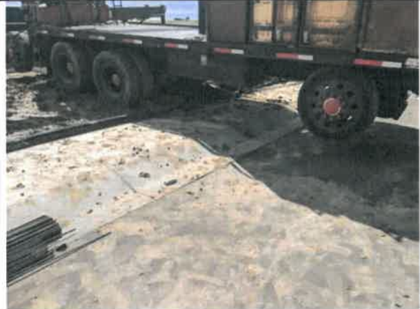
Image 4 – Damaged concrete and settled asphalt in vicinity of home construction. Typical in areas around site.
