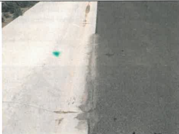
Image 5 – Previous patching is cracking at the connection and overlap of asphalt paving.
