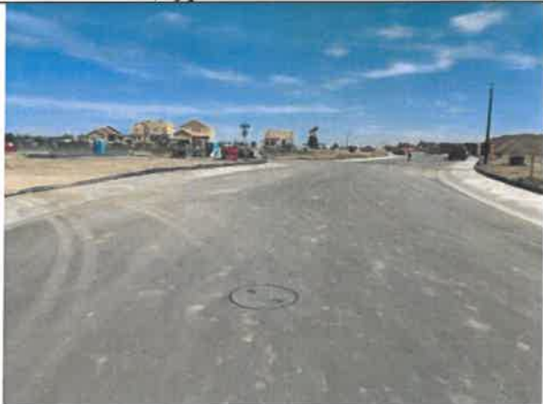
Image 17 – Settling of asphalt within Jersey Drive.
