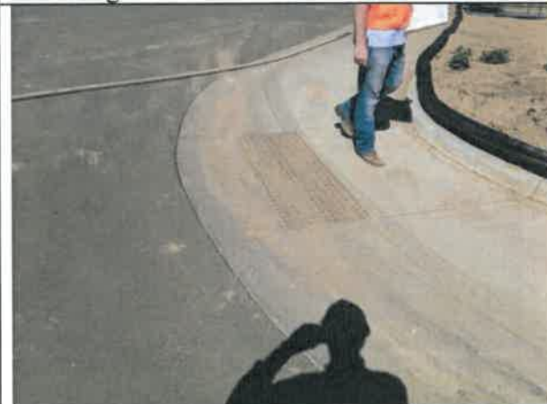
Image 14 – Settled asphalt, and asphalt pulling away from curb and gutter at the northwest corner of the Angus Street and Longhorn Drive intersection.
