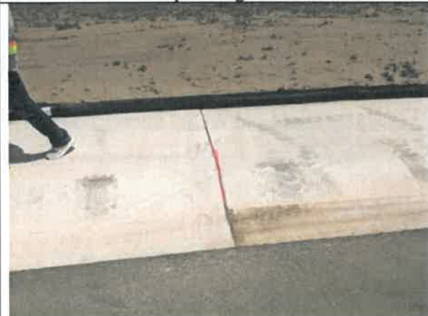
Image 8 – Concrete flatwork has settled, and expanded openings of control joints shown. Typical in areas around site.
