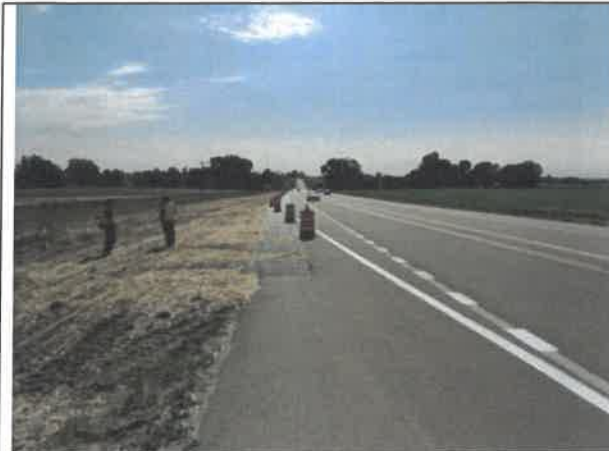
Image 3 – Delineators along Highway 66 not installed, and taper and dashed striping west of WCR 5 does not meet permit documents.
