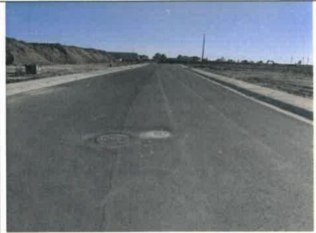
Image 2 – Settled SSMH, valve color, and asphalt within Longhorn Drive, and typical in site areas.
