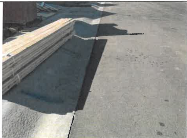
Image 7 – Settled asphalt along gutter, stained asphalt, and damaged concrete observed within Longhorn Drive.
