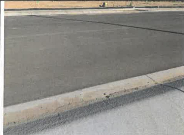
Image 5 – Asphalt edge extends to far above adjacent concrete edge, and damage to edge of concrete gutter.
