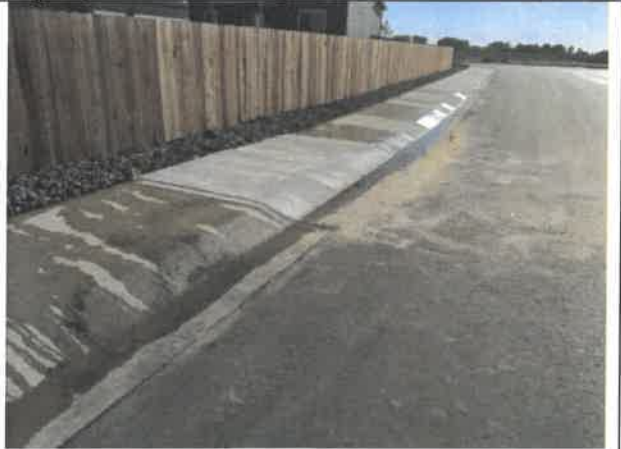
Image 6 – Water from adjacent dwelling site is overflowing from Block 12 Lot 8 to right-of-way flatwork along Gelbvieh Street causing staining along concrete.
