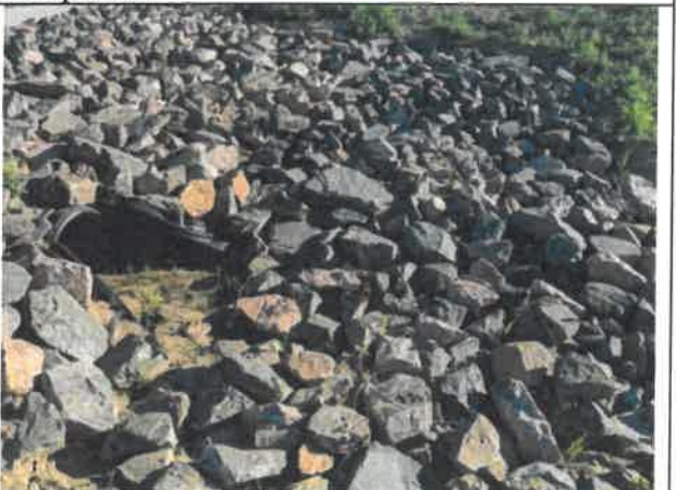
Image 8 – Riprap placed above FES invert out is trapping sediment.
