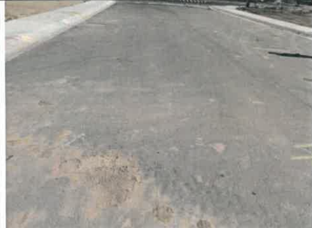
Image 12 – Asphalt cores, damaged asphalt, and settling asphalt observed within Longhorn Drive from Angus Street to WCR32.
