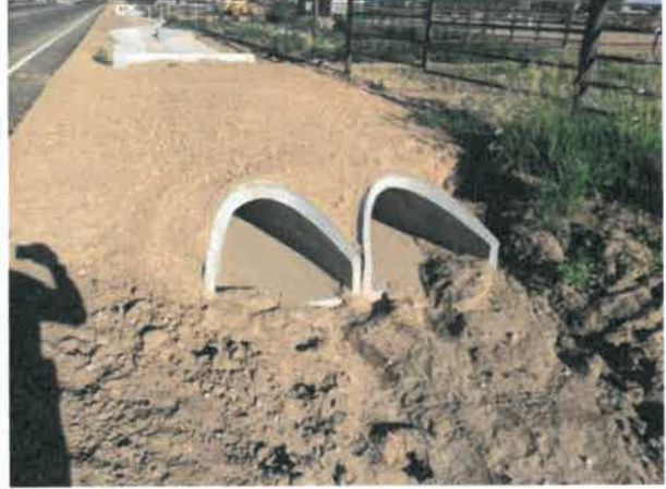
Image 10 – Riprap not provided at double FES per Town standards.
