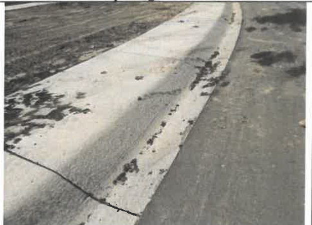
Image 6 – Aesthetic damage to concrete curb & gutter, typical in areas around site.
