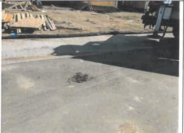
Image 8 – Damaged asphalt, typical in areas around site.
