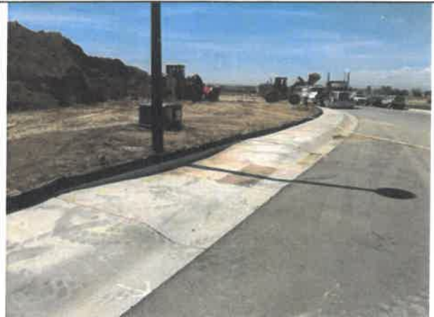
Image 16 – Concrete tie-ins have greater than ¼” vertical threshold providing a trip hazard, typical in areas around site.
