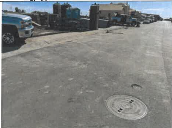
Image 7 – Asphalt settling, and gate valve cover too low observed within Angus Street
