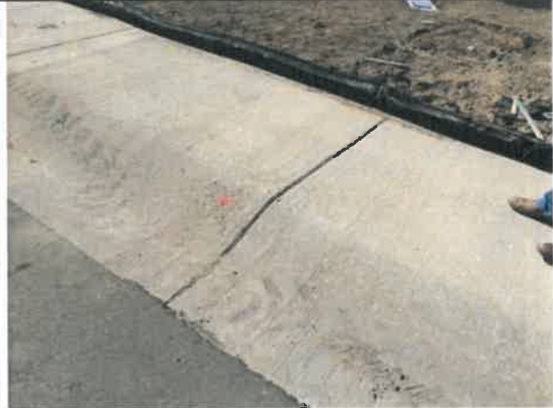
Image 10 – Poor concrete finishing workmanship observed, typical in areas around site.
