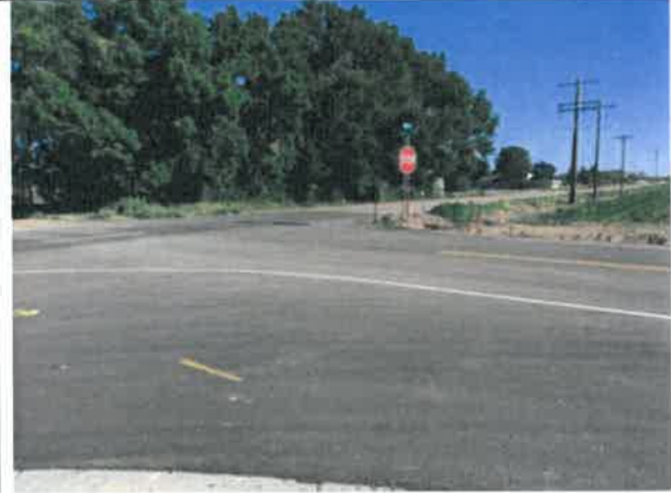
Image 12 – Stop bar along WCR 32 at WCR 5 intersection missing, typical both sides.
