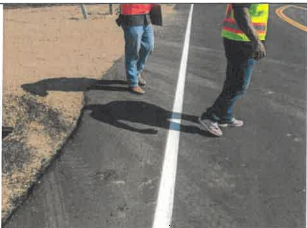
Image 7 – Damage to installed asphalt along WCR 5.
