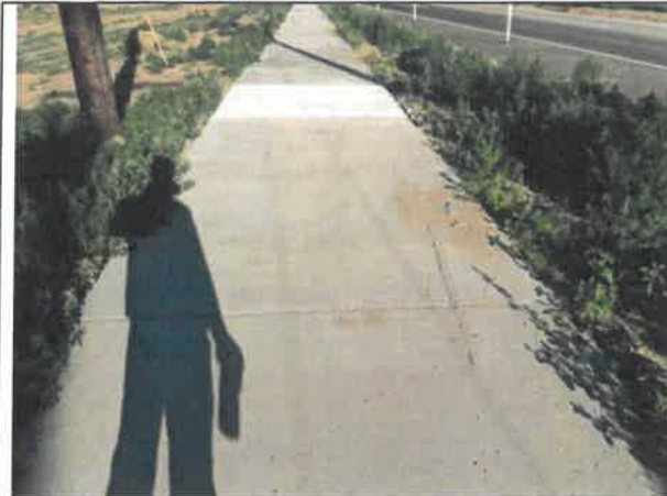
Image 3 – Excess concrete caked onto to walk surface.
