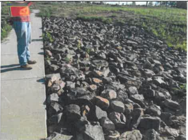
Image 7 – Gaps and holes along concrete walk in spillway area pose a trip and injury hazard.
