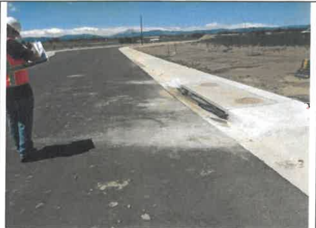
Image 10 – Concrete splatter observed, settlement/compression of asphalt, and evidence of ponding water / settled concrete. Typical in areas around site.
