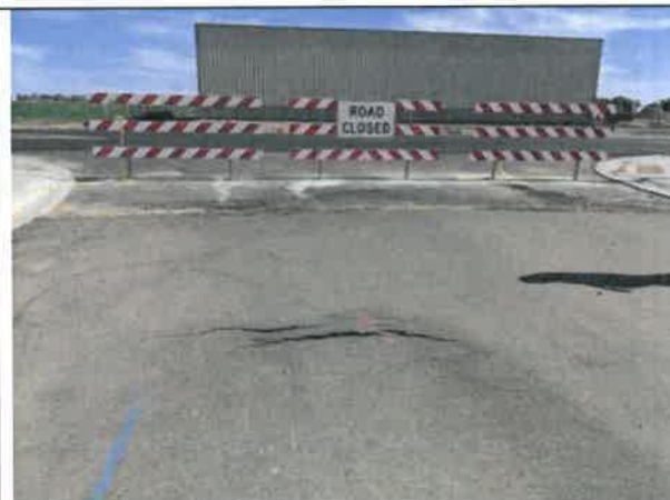
Image 13 – Damaged asphalt within Longhorn Drive near the intersection of WCR32
