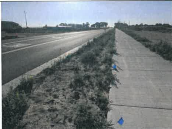
Image 1 – Landscape area between concrete walk and back of curb does not have positive drainage. Chipped and damaged concrete observed, typical in areas along WCR 32.
