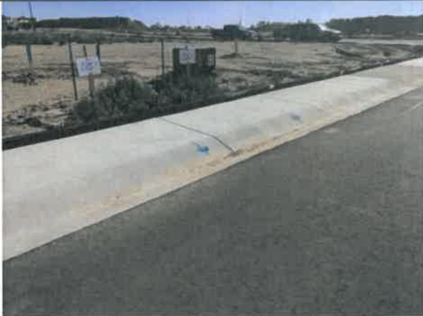
Image 9 – Concrete pan along Gelbvieh Street trapping stormwater and depositing sediment.
