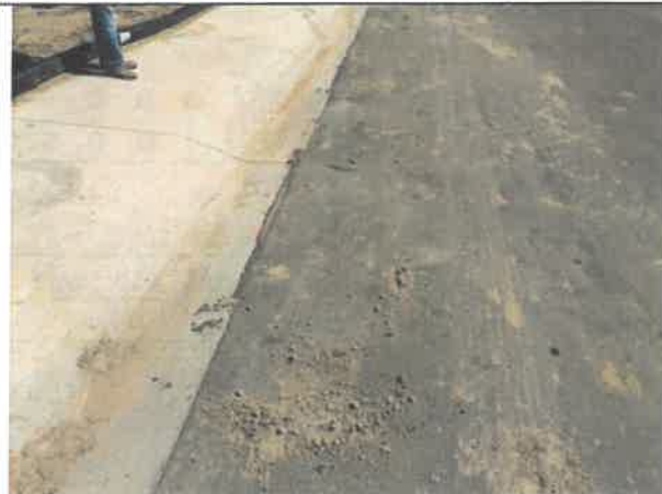
Image 15 – Excess asphalt over concrete surfacing, and dirt/sediment within stormwater infrastructure, typical in areas around site.
