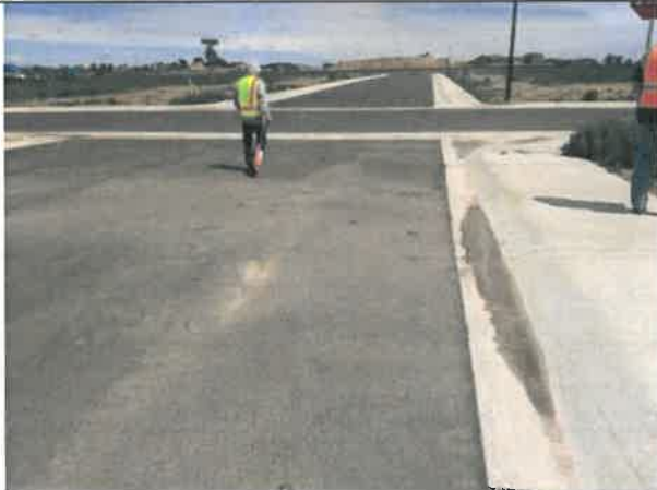
Image 3 – Concrete flatwork is ponding water, asphalt placed over concrete, and compressed asphalt is holding sediment/water. Typical in areas around site.
