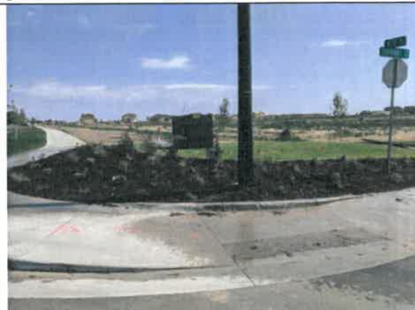
Image 13 – Curb ramp at WCR 5 and Charbray Street does not meet ADA accessibility.
