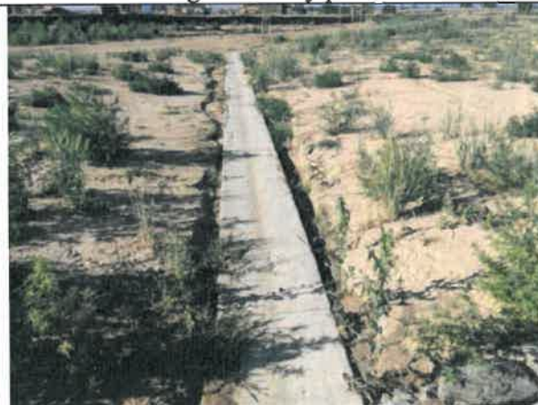
Image 13 – Soil materials eroded along concrete pan preventing runoff from reaching pan flowline. Typical in site areas throughout.
