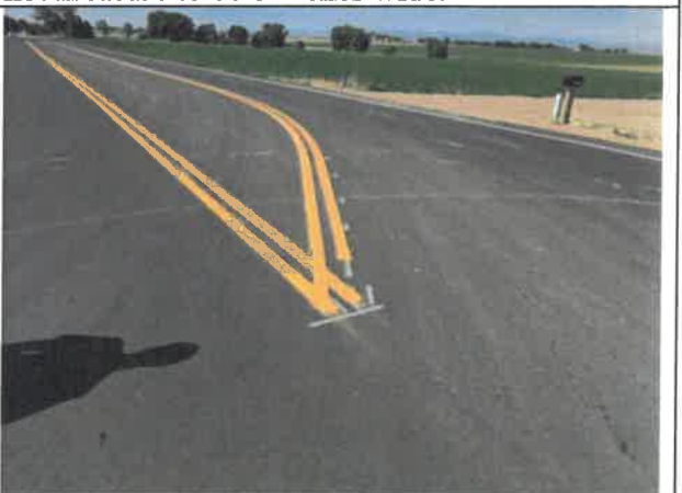
Image 8 – Double striping not connected within WCR 5 at Charbray Street.
