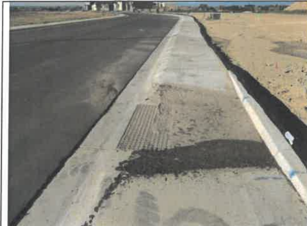
Image 3 – Accumulated debris within curb ramp, typical in areas around site.
