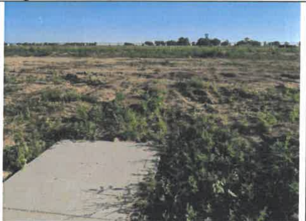
Image 6 – Concrete walk connection from the rip rap spillway to WCR 32 detached walk not completed.
