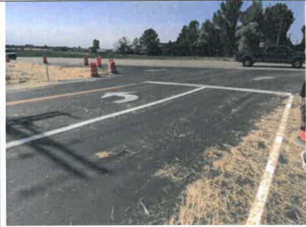
Image 2 – Lane widths at the intersection of WCR 5 and Highway 66 do not measure to be 12-foot wide. Measurements range from 10'-8" to 11'-8". Shoulder widths measure greater than 4-foot wide.
