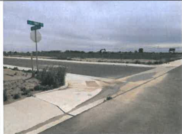
Image 6 – Concrete flatwork and intersection cross pan at intersection of Galloway Street and Shorthorn Drive is ponding water.
