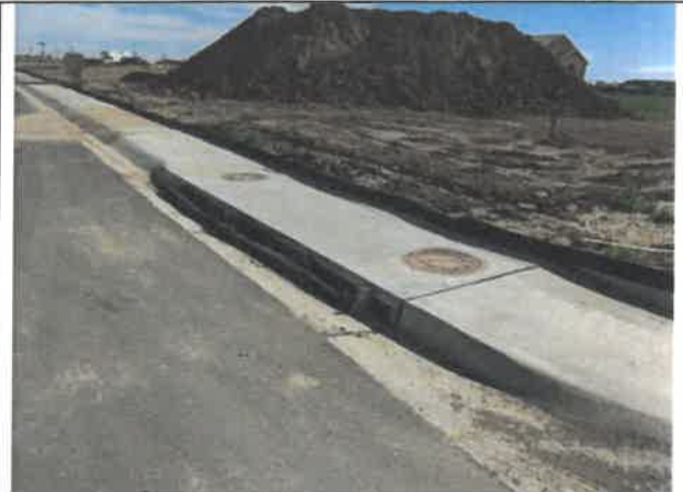
Image 4 – Rock sock across throat opening does not cover entire opening.
