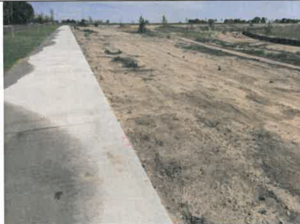
Image 11 – Chipped concrete walk along WCR 5
