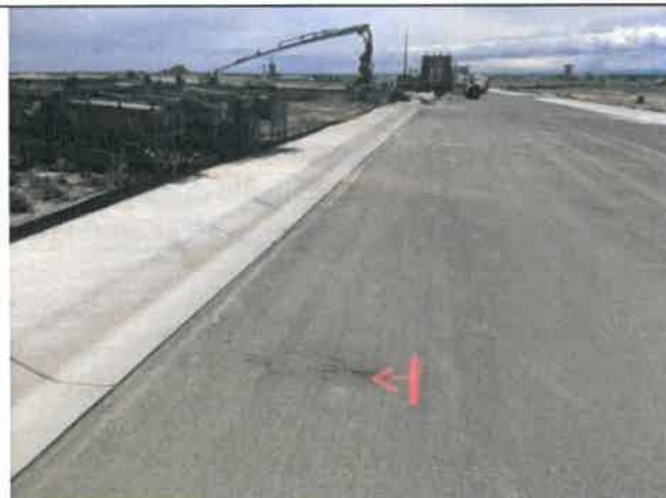
Image 7 – Slippage cracks. Typical in areas around site.
