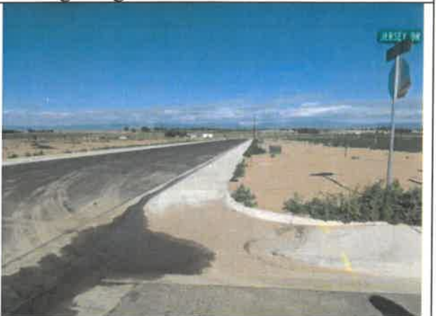
Image 8 – Accumulated sediment, and a low spot observed in the concrete pan at the Jersey Drive and Gelbvieh Street intersection.
