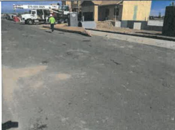
Image 9 – Settling of asphalt around manhole and gate valve cover, stained asphalt, scuff marks, and damaged asphalt within Angus St.
