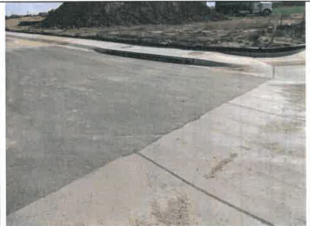
Image 2 – Gouged asphalt, typical in areas around site.
