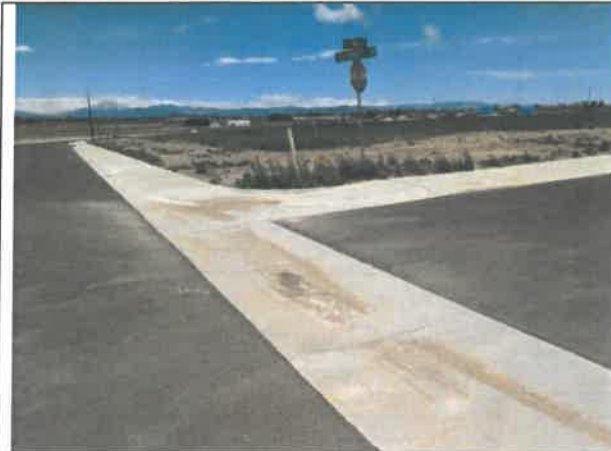
Image 9 – Concrete flatwork and intersection cross pan at intersection of Galloway Street and Piedmontese Drive is ponding water. Concrete gutter along Galloway has settled trapping sediment.
