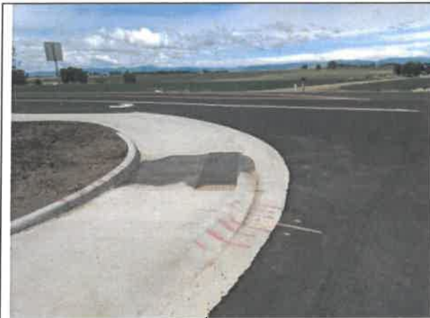
Image 1 – The southeast curb ramp at the Charbray Street and WCR5 intersection is holding water.
