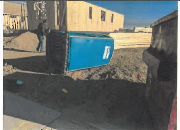
Image 4 – Wind from previous weekend’s storm event has caused blown debris, and tipped port-o-pottys.
