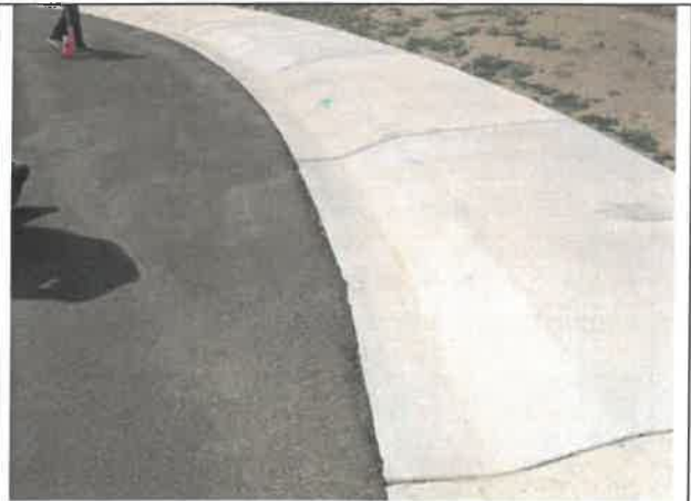
Image 2 – Gaps observed between asphalt and edge of concrete, and aesthetic damage to concrete surfacing. Typical in areas around site.
