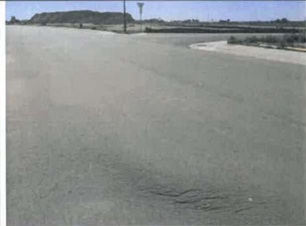
Image 12 – Slippage damage to asphalt observed with Charbray Street. Typical in areas around site, with more instances showing over time.
