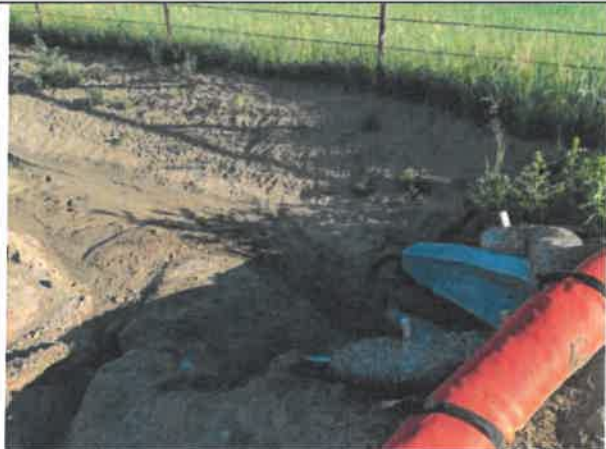
Image 5 – Unstabilized soils showing signs of erosion, riprap for FES missing at FES along north portion of WCR 32.
