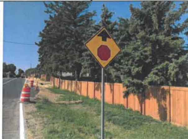
Image 5 – Stop sign not installed in the location per Permit Documents
