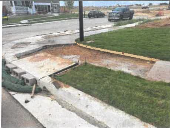
Concrete Item (Hole was full of water)
