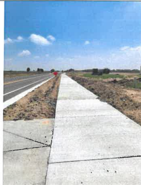
Concrete Backfill not done for over a month
