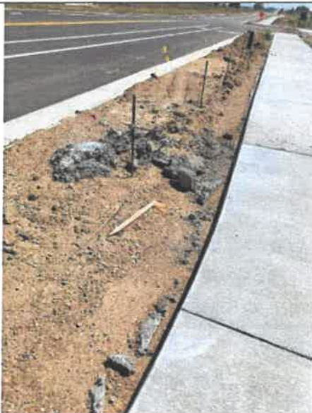
Concrete (Damaged) Backfill not done for over a month
