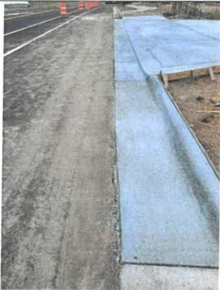
Concrete (Clean up and curb not tapered to zero) Backfill/Cleanup
