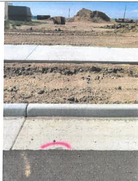
Concrete (Damaged) Backfill not done for over a month
